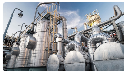
Chemical and Process Technology - Aerzen
